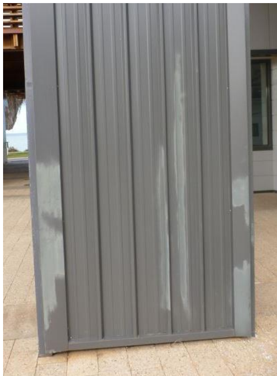
Fig 1: Colorbond wall cladding damaged by a corrosive atmosphere.
